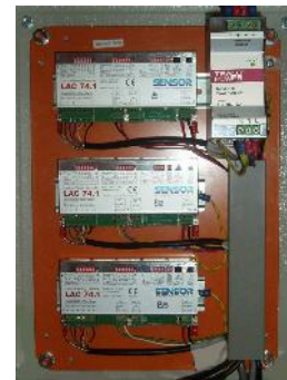
Loadcell Amplifier Cabinet
